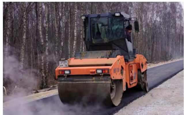
Figure 6: Roller in Russia implementing the MCA-2000 control system
