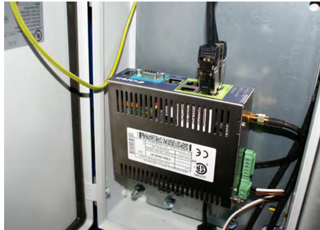
Figure 1: The Ewon router was installed in a small cupboard next to the actual control cabinet; not for technical reasons, but because of the shape of the switchboard; this solution proved to be more economical than a bigger control cabinet
